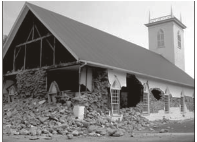
Kalahikiola Congregational UCC in Kohala, Hawaii, sustained severe damage during the Oct. 15 earthquake.
